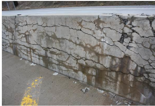
Figure 1.2. Example of ASR symptoms such as map cracking, cracks parallel to restraint, gel exudation, and surface discoloration. Picture used with permission from Richard Deschenes.
