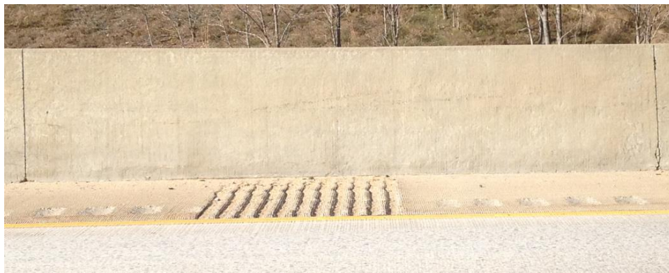
Figure 2.1. A median barrier section which exhibits minimal damage, (e.g. 3no visible map cracking). Picture used with permission from Richard Deschenes.
